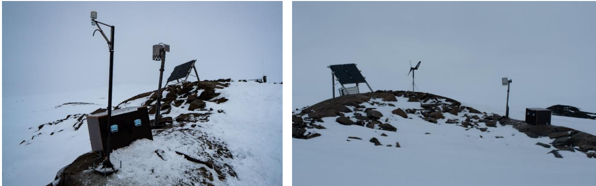
Figure 2: View of the installation at the CLIMB remote site; left image, from left to right: the pole with the meteorological data logger and the inlet for the optical particle sizer (OPS) attached to it; below the box with the OPS inside and other controlling devices for the VOC sampler and power control, in the middle the pole with the VOC sampler and the solar panel; right image: the wind turbine can be seen and another power-control-battery box under the solar panel
