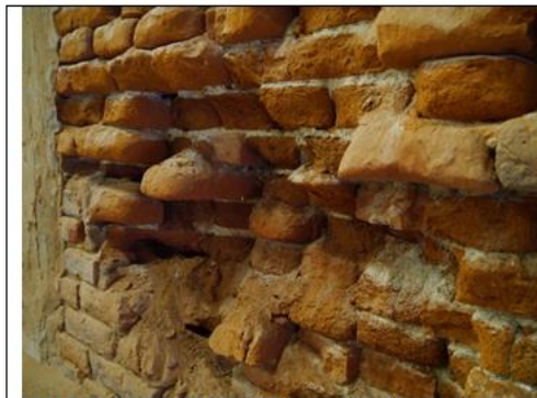
Figure 1. Example of salt damage to historic masonry (Photo KIK-IRPA, Hof te Bree-Eik)
