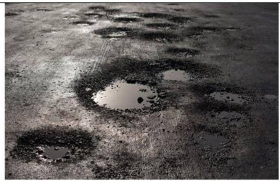
Figure 2. Example of salt damage to roads and bridges (Photo via Shutterstock)
