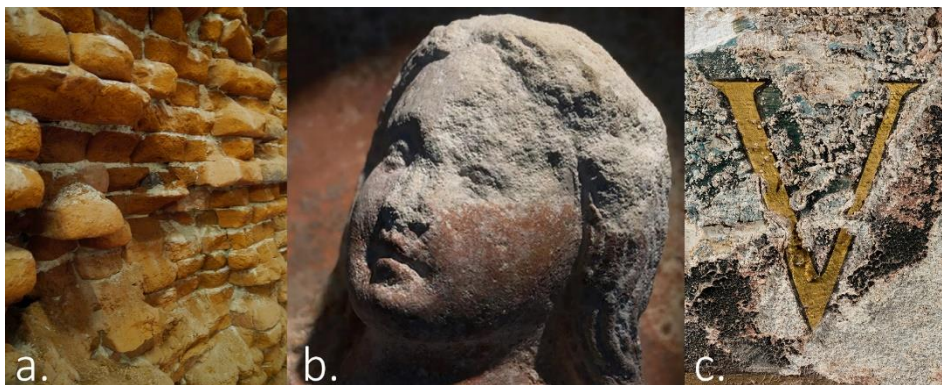
Fig. 0.1 Examples of salt-related deterioration of (a.) 17th-century brick masonry of the Farm Bree-Eik (Lennik, Belgium), (b.) 15th-century limestone (Avenderstone) sculpture in the Church of Saint-Martin (Hainaut, Belgium), and (c.) 18th-century mural on limestone plaster in the Church of Sint-Aldegondis (Mespelare, Belgium).
